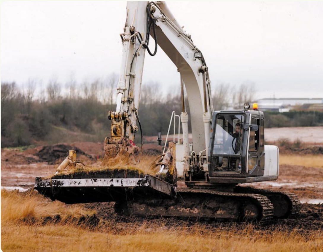
Turves of valuable ancient wet heathland being lifted in their entirety at Norton Canes
